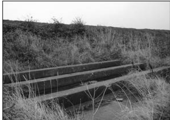
Supports for fuel tanks.
